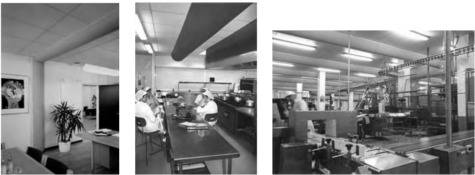
Figure 5.25 Some applications of textile ventilation ducts (courtesy of KE Fibertec).
